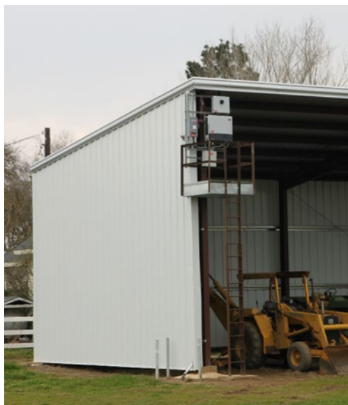
Figure 25: Elevated Electric Service and Equipment
